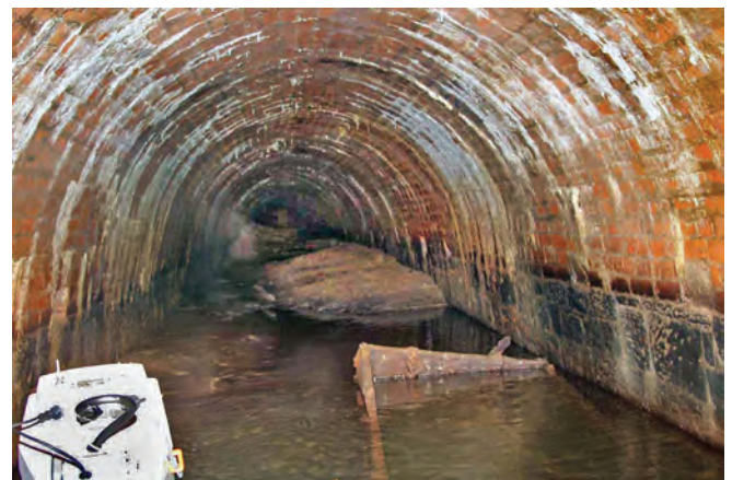
The tunnel is navigable for 440 metres. Beyond that the tunnel is blocked by a sunken pan; beyond that the first roof fall is soon reached. Photo John Lower
